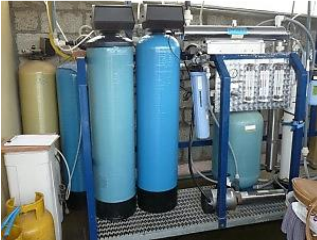
Reverse osmosis purification system is the process to clean water.
