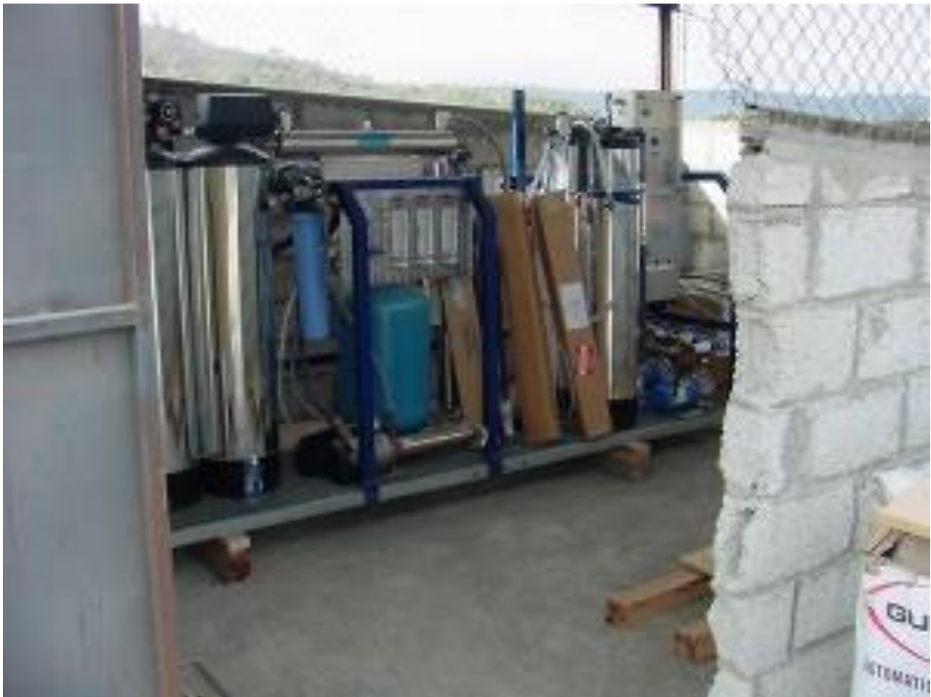
Water purification system
