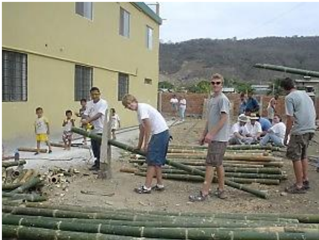
Construction team working with bamboo poles, which are used to support the construction of a roof/ceiling
